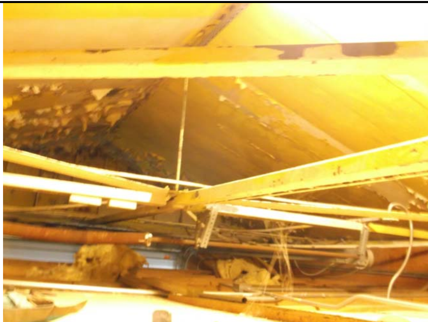
Photo 2: View of the lead-based paint (white & yellow) observed in the attic of the Bos'n Hole building.
