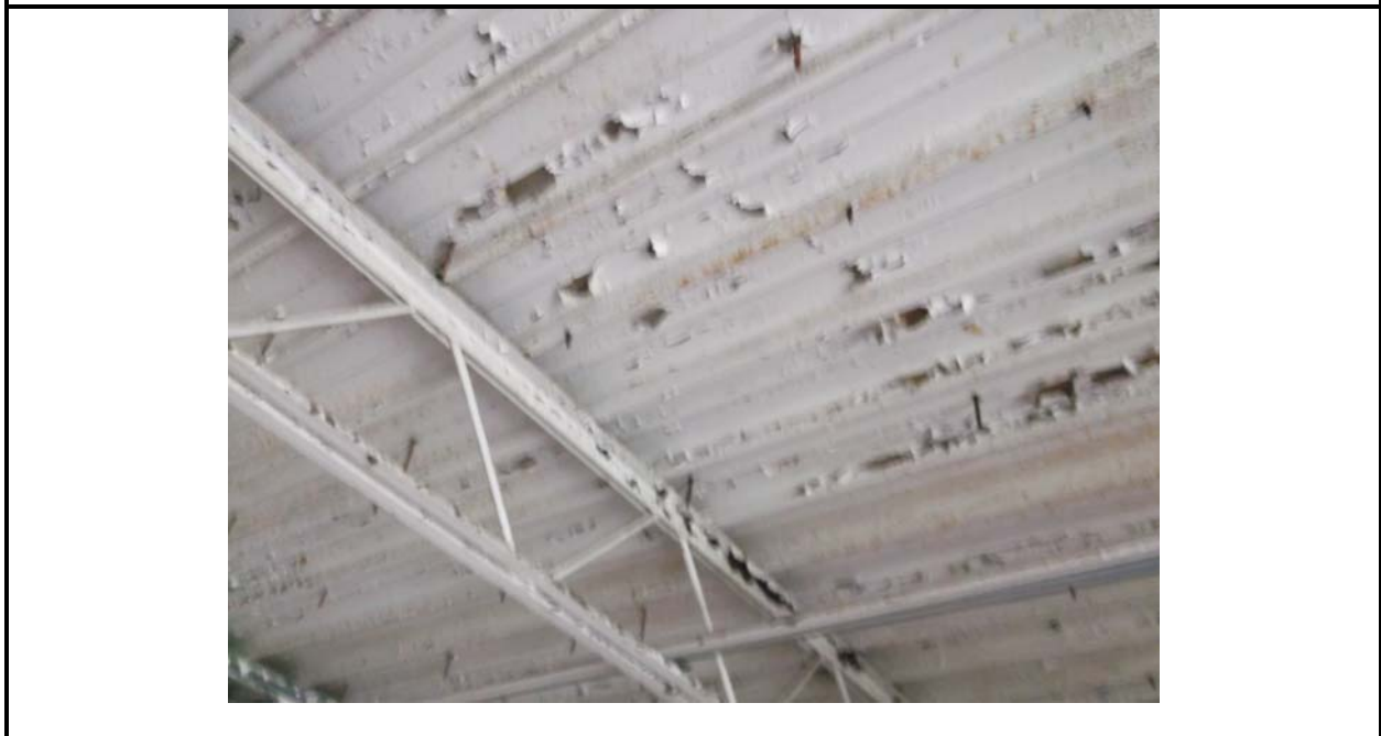
Photo 4: Heavy peeling observed of the interior paint on the exposed metal deck roofing of the DC Shop (OS1).
